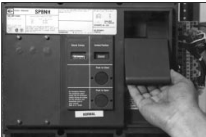
Figure 5-1 Pumping Handle Charges Stored Energy Mechanism
